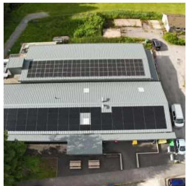
The new solar panels at the front of the building double the amount of electricity we can generate.
